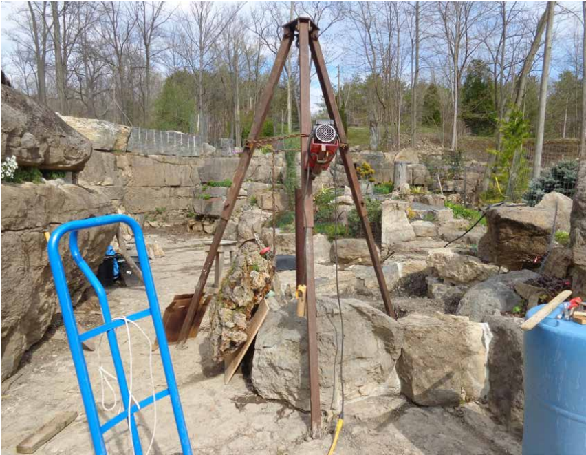
Top: Lifting a tufa slab into place with a tripod and electric winch.
