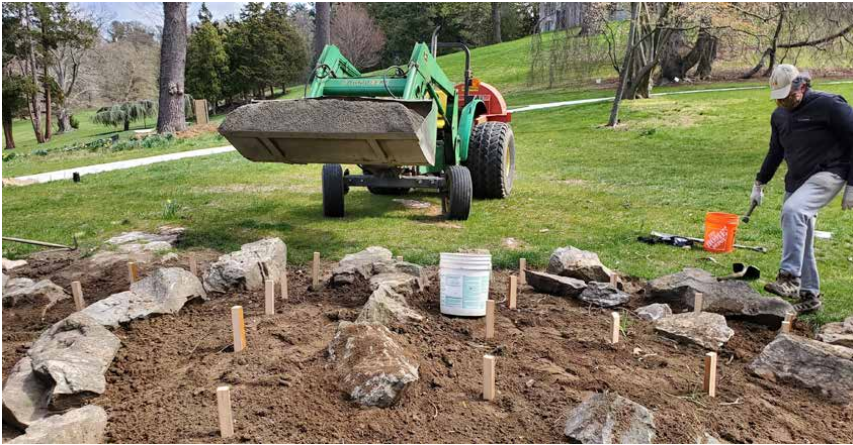
Rocks going into place (top) and applying a layer of sand over the soil (bottom)
