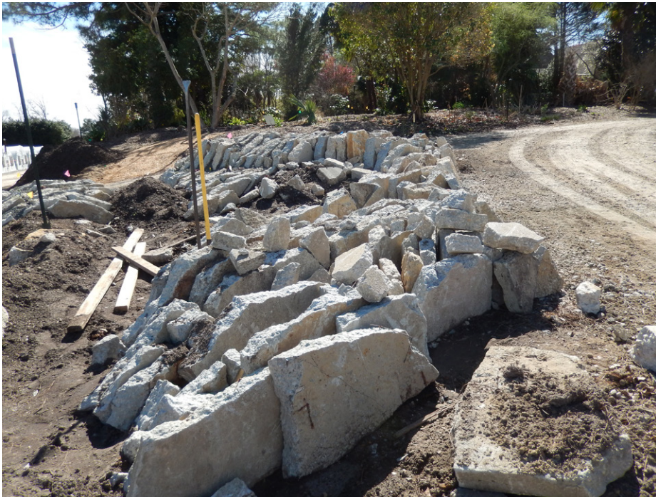
Crevices under construction.
